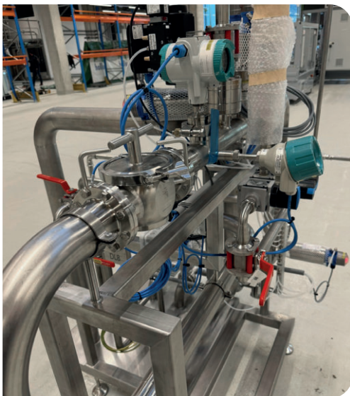
Pig station for catching and returning pigs in ATEX design in a cleaning agent production plant
